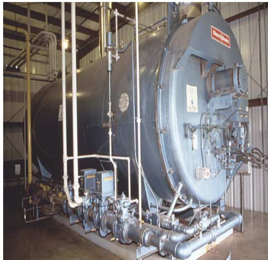
Cleaver Brooks 20,000 lb/hr Boiler
