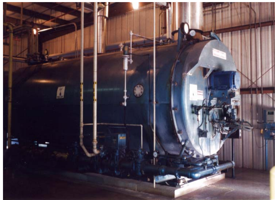
Cleaver Brooks Boiler Unit
