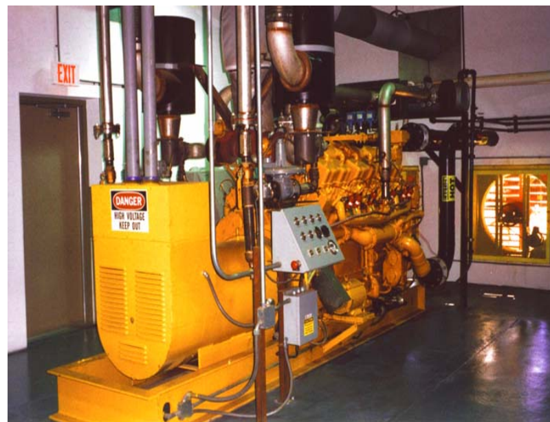
Caterpillar 3516 800 kW Genset
