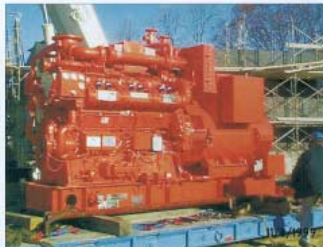
The engine was set in place at the Nashua wastewater treatment plant and a brick structure was built around it.
