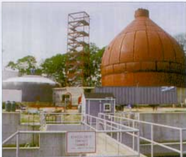
The egg-shaped digester, where methane gas is produced, is a new concept in the U.S. but has been used in Europe for 25 years.
