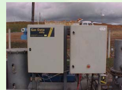
Painel de Controle
