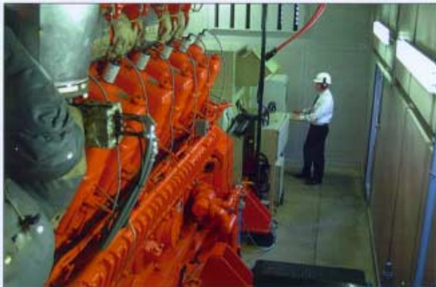
The engine provides 2.5 MW of power plus heat for process water and to run absorption chillers.
